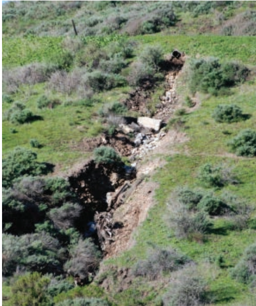
BEFORE: Erosion resulting from improperly designed drainage system
