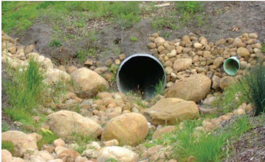
Rip rap drainage system
