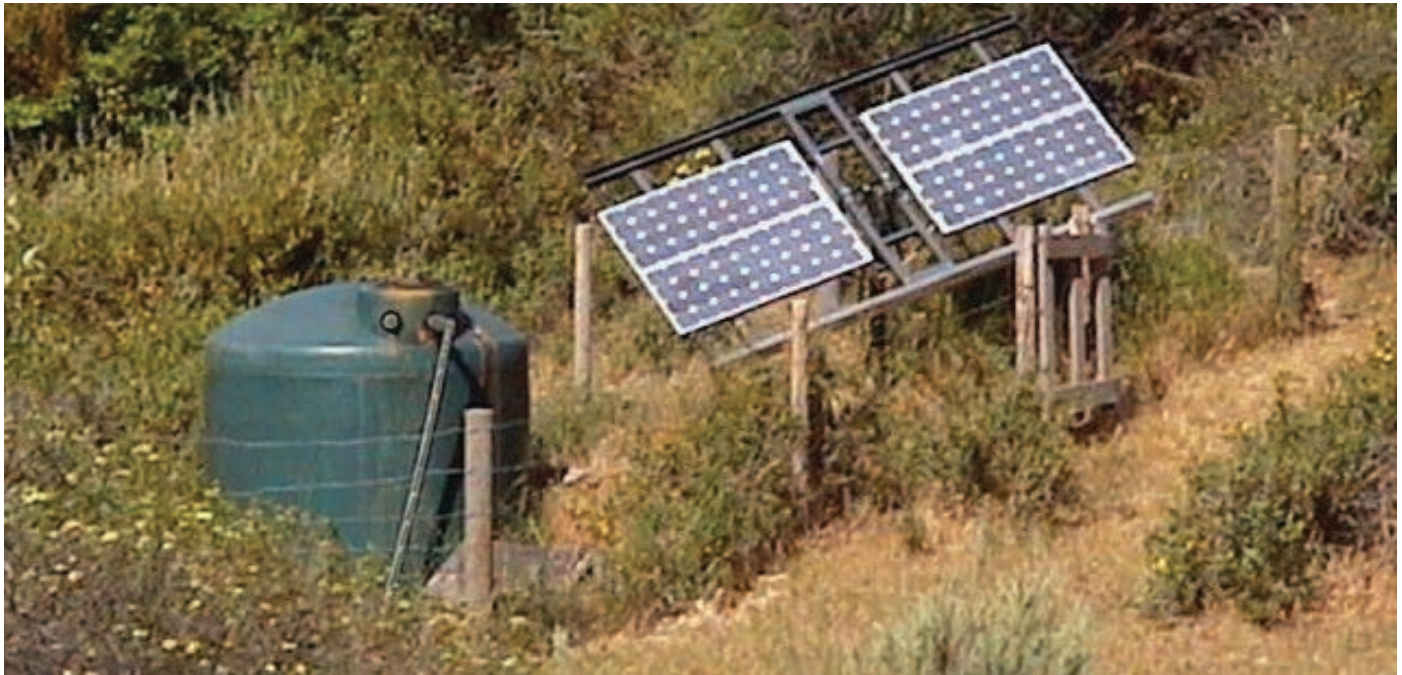
Photovoltaic panels and water storage
